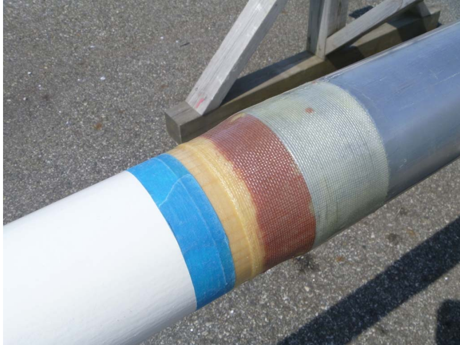
13. Mai, The joint has just been glassed and will later be painted with 2-pot paint. The top section was not glassed, just painted with 2-pot paint as well.
